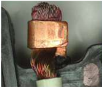
▲ Multiple wires and a terminal
